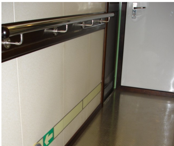
Figure 2. Marking of egress path with photoluminescent strips
