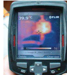
Fig. 26. Proper working pump
