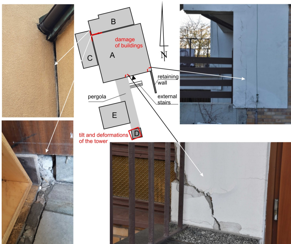
Figure 8. Damage and deformation observed in buildings
