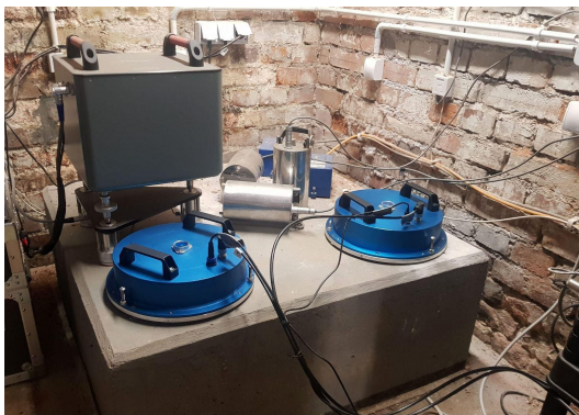
Fig. 5. General view of FOS5-01 and FOS5-02 installed at seismological platform together with another seismological device for measurements in the “Ignacy” coalmine in Rybnik.
