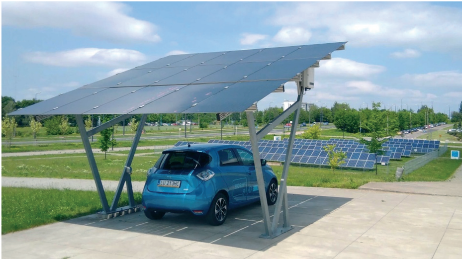
Fig. 6. Photovoltaic installation in the form of a carport (foreground) and placed on the ground (second plan)
