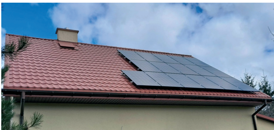
Fig. 5. Photovoltaic installation placed on the roof of a residential building
