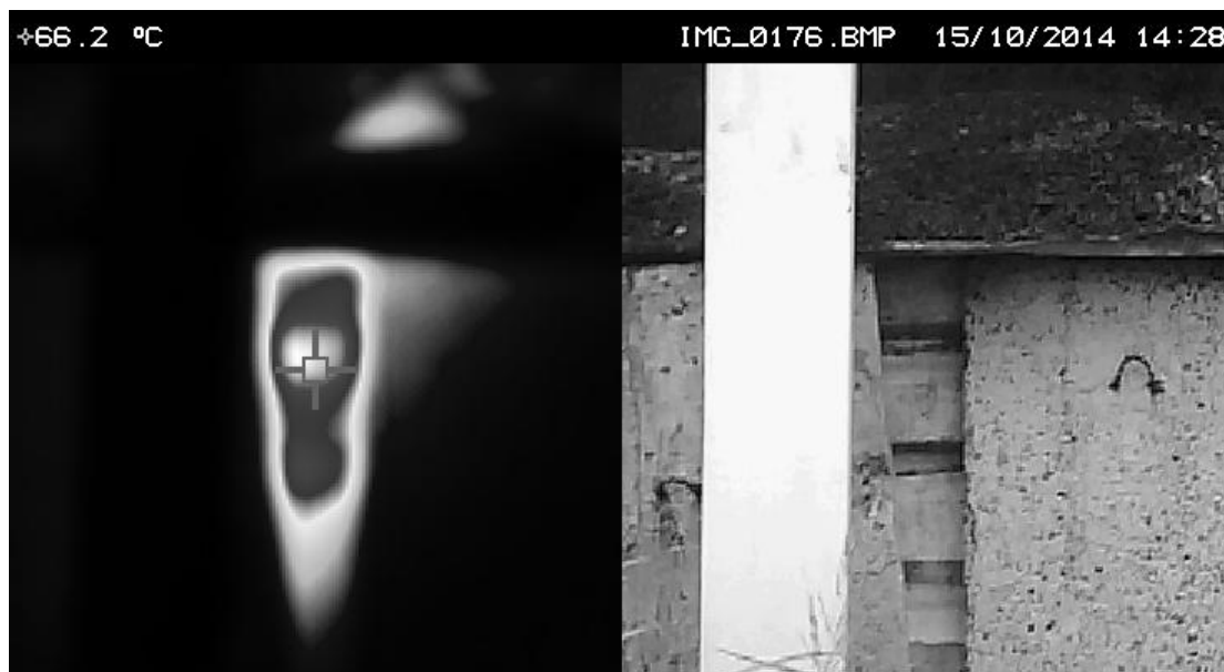
Fig.4. Thermal image indicating the rise of temperature of stored coal in place of damaged retaining wall (Author: Bogdan Sobociński)
