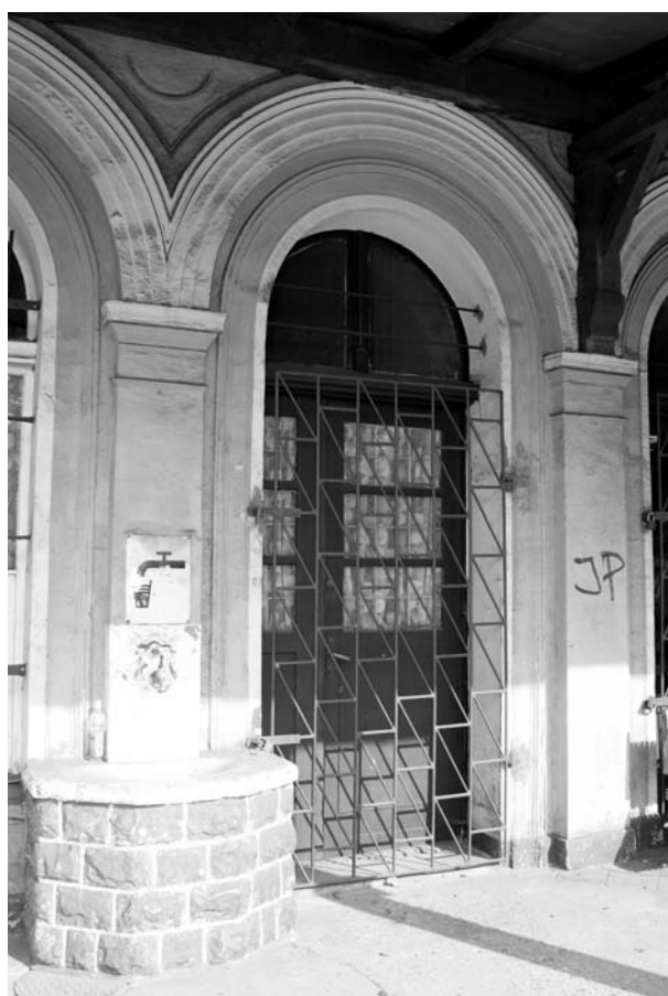
Fig. 3. Fragment of classical finishing of the wall of the station in Gogolin. Simple classical pilasters and arches are modelled on the Doric order. The rafter framing of the shed and the tap were added later (Pic. by author, 2009).
