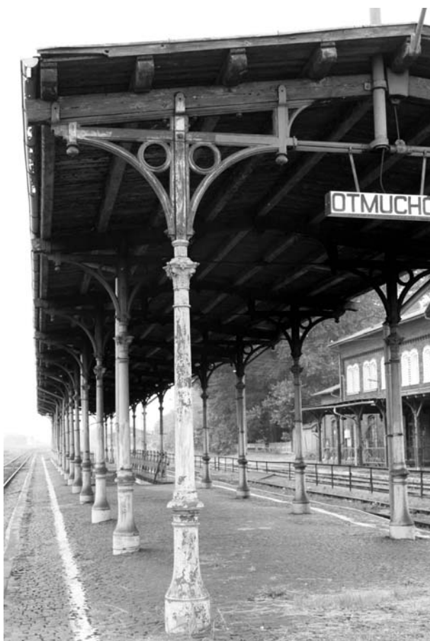
Fig. 2. A shed of the island platform in the station in Otmuchów. Cast-iron decorative poles carry steel trusses on which the wooden rafter framing was based. Clearly one can see the classical tripartite division of the pole modelled on the Corinthian order (Pic. by author, 2009).
