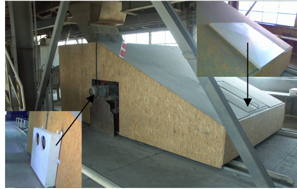
Fig. 10. Realized sound insulating enclosure
