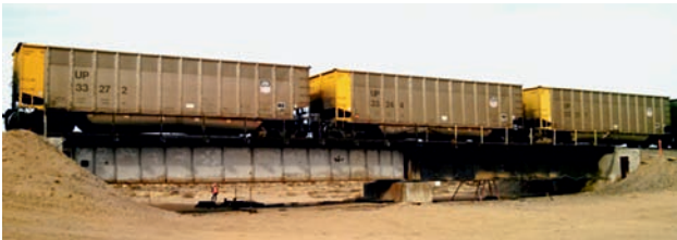
Fig. 9. One of the bridges at the FAST testing ground in Pueblo [source: TTC]
