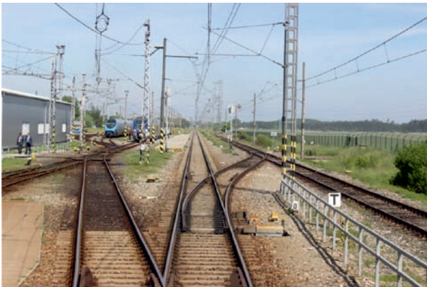
Fig. 7. VUZ test circuit in Velim – straight section with turnouts and technical station [photo by A. Massel]
