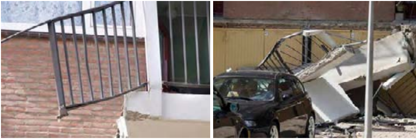
Fig. 9. Unannounced collapse of gallery plates in an apartment building in Leeuwarden, The Netherlands, 2003
