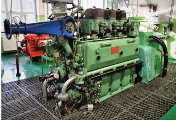
Fig. 1. Photo of the SULZER 3AL25/30 piston engine facility [7]
