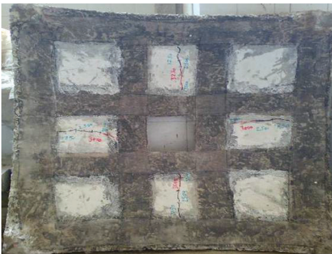
Fig. 21. Crack pattern of shell Strengthened by using 2 layers GFRP (Type 2). [Failure load = 3500 kg]
