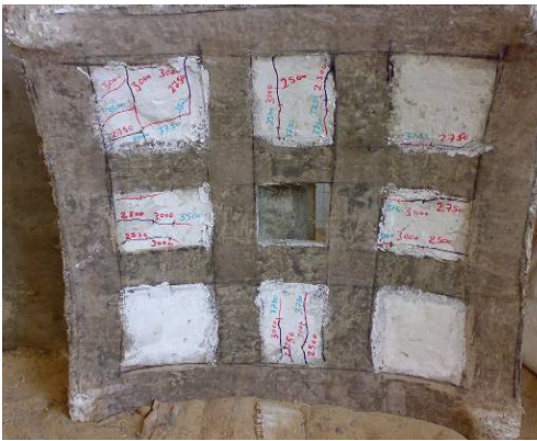
Fig. 25. Crack pattern of shell repaired by using 2 layers GFRP (Type 2). [Failure load = 3750 kg]
