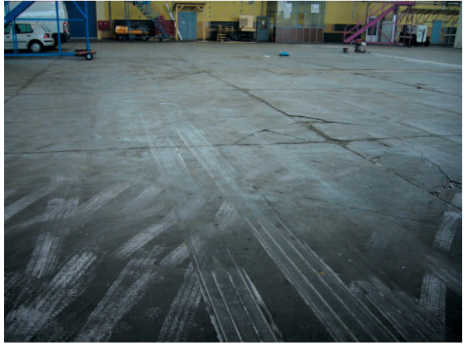
Fig. 2. The hangar slab with visible damages
