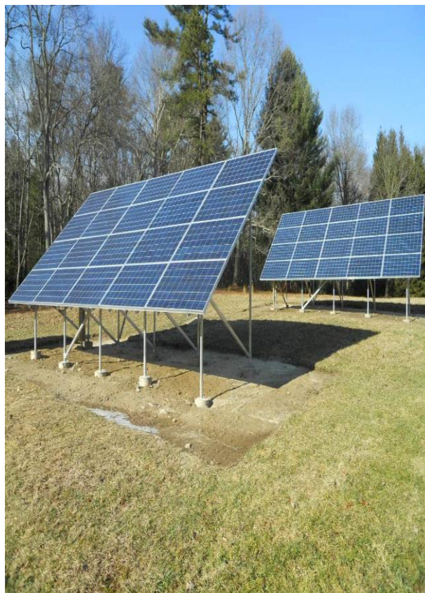
Figure 3: A solar garden array ( https://www.sunshinecoast.evolutionsolar.com.au )
