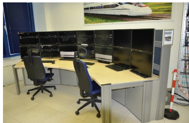
Fig. 4. Traffic safety system test stand at the Bombardier ZWUS plant in Katowice [photo M. Graff, 30.05.2017]
