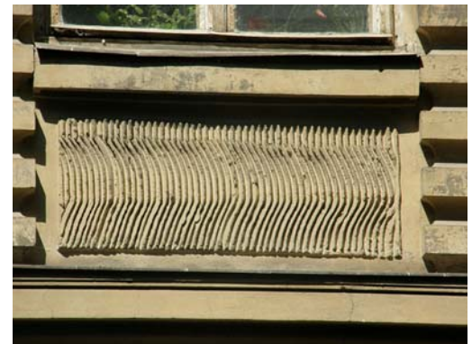
Fig. 30. Molding with plaster texture (14 Dontsova str.). Source: il. T. Kazantseva, S. Ponkalo
