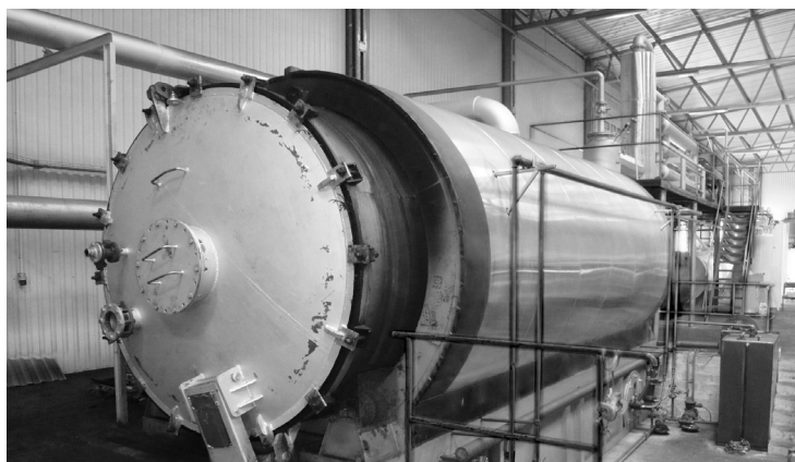
Fig. 1. Discontinuous pyrolysis plant XY-8 (batch process) of company Shangqiu Jinpeng Industrial Co., Ltd. – reactor or rather rotary pyrolysis kiln (photo – author)
