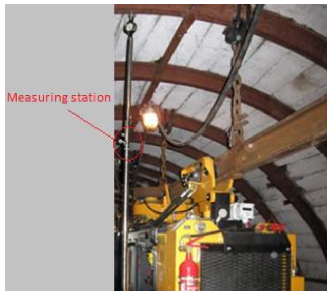
Fig. 2. Measuring station for recording the deformations of arch fastening during transportation of heavy loads
