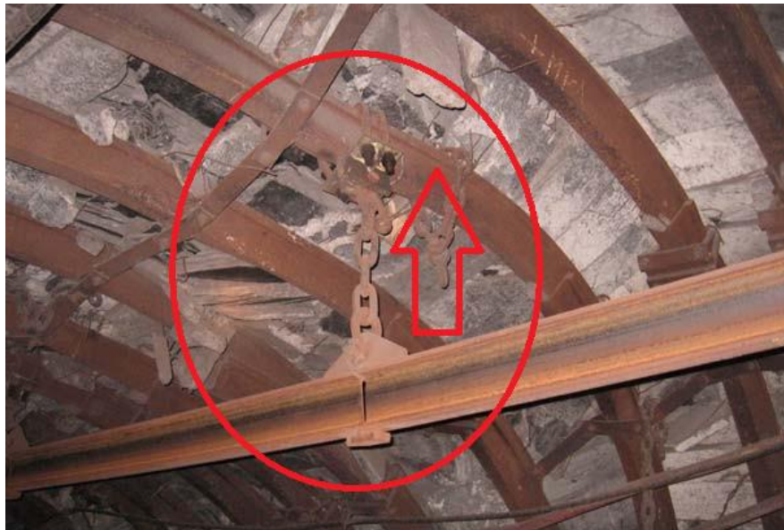
Fig. 1. Mechanical failure due to dynamic loads and local deformation of the roof
