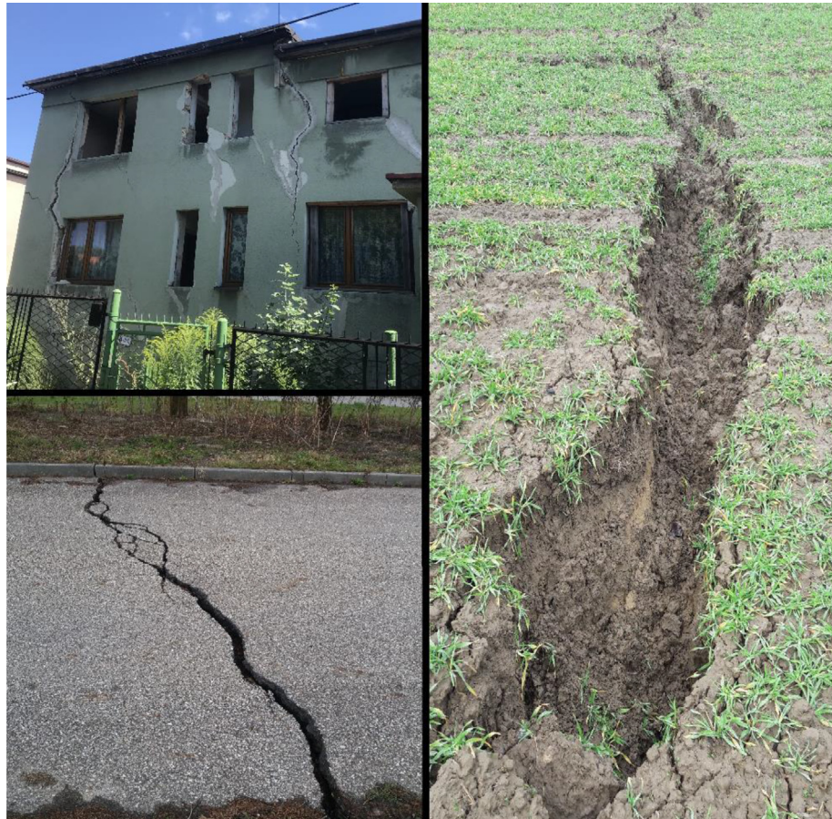
Fig. 1. Examples of linear discontinuous ground deformations (LDGDs).
