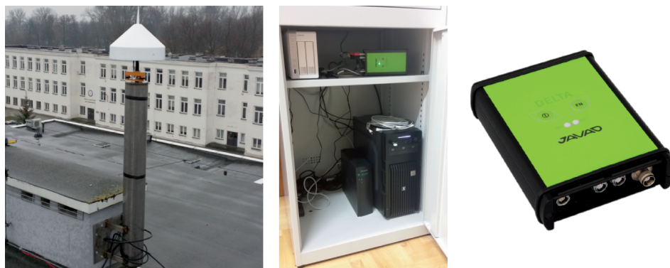
Fig. 2. Equipment of permanent GNSS monitoring station in Dęblin
