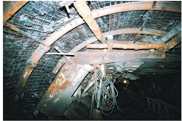
Fig. 7. Longwall equipment, development drift driven in coupled ŁPK frames
