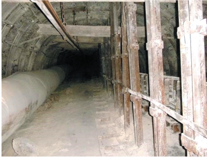
Fig. 16. Development drift secured by means of the ŁPKO support
