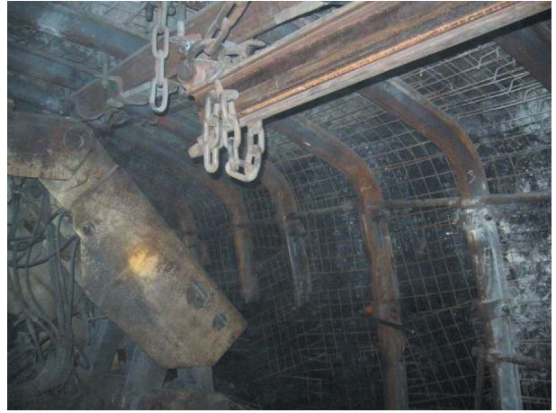
Fig. 34. Longwall equipment, development drift secured with four-element ŁPrP frames
