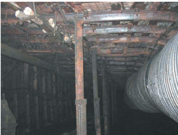
Fig. 19. Development drift secured by means of the ŁPro/B support
