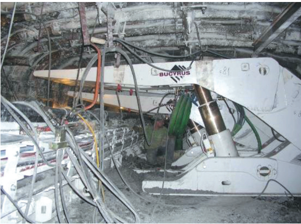
Fig. 41. Longwall equipment in a development drift secured by means of the ŁPrP variant K support
