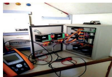
Fig. 11. PQ analyzer connected to extract the data
