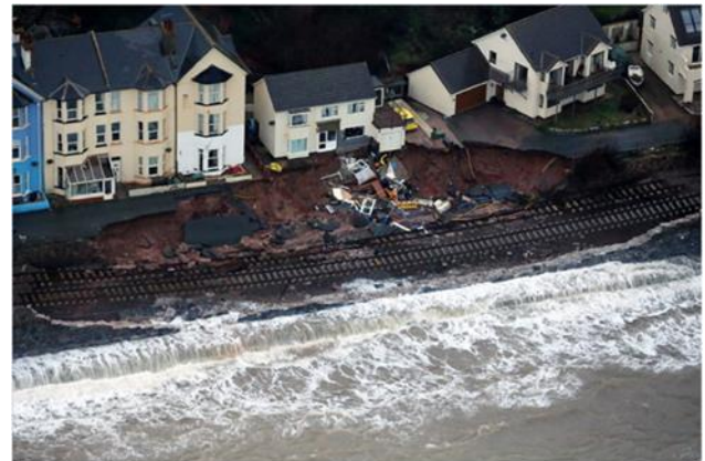
Figure 2. The breach in the sea wall near King Harry's Walk at Dawlish, Devon, on 7 February 2014
