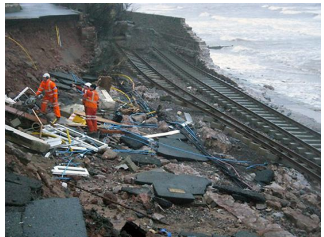
Figure 3. Investigation of the damages according to [26]
