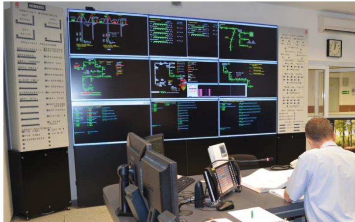
Fig. 4. Tauron's control room [7]
