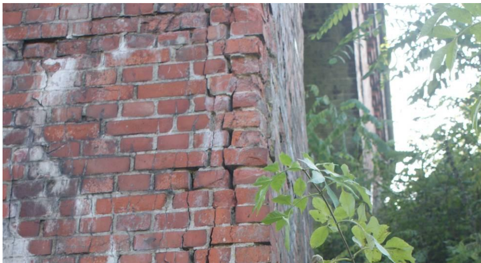
Fig. 7. View of viaduct pillar B. Visible cutting of the outer layer of bricks
