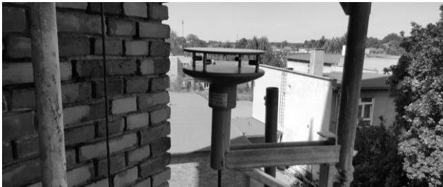
Rys. 5. Anemometry 2D pomiędzy słupkami rusztowania Fig. 5. 2D anemometers mounted between scaffolding standards
