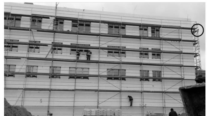
Rys. 8. Widok rusztowania w Krośnie z anemometrami Fig. 8. The view of a scaffolding in Krosno with anemometers
