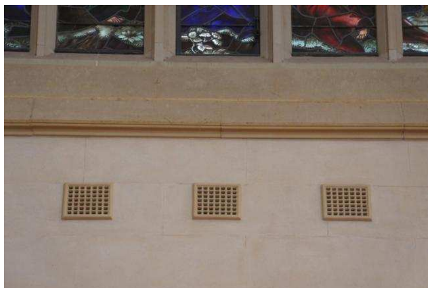
Fig. 8. Detail of the elements of the ventilation system - exhaust grilles. Visible effect of properly chosen elements to the historic character of the cathedral interior
