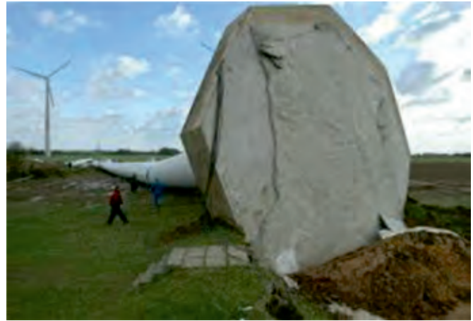
Fig. 2. Failure of wind turbine foundation [1]
