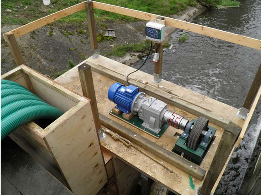
Fig. 4. Electricity generation section with electrical system elements [Włodzimierz Sawicki, 2010]
