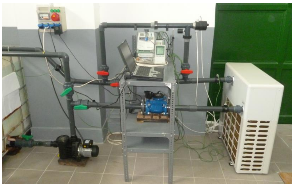
Fig. 3. Heat pump measurement circle at Szent István University, Faculty of Mechanical Engineering
