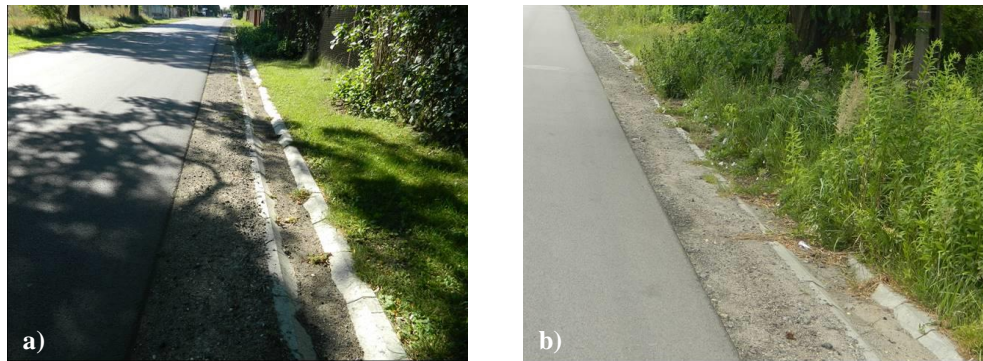
Fig. 6. Incorrect positioning of an oval gutter: a) shortly after construction, b) after two years
