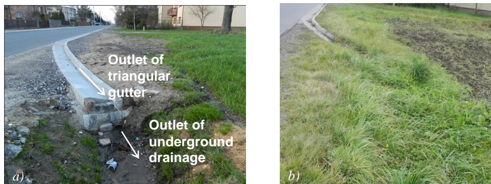
Fig. 9. Loss of dewatering functionality due to lack of maintenance: a) drainage elements one year after construction, b) after three years
