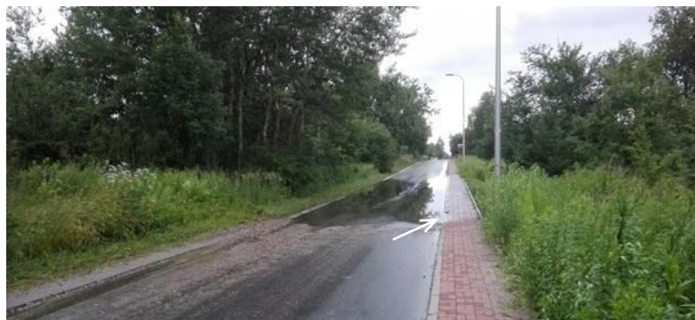
Fig. 10. Deposition of rainwater in a lowering of the area, clogged drainage inlet
