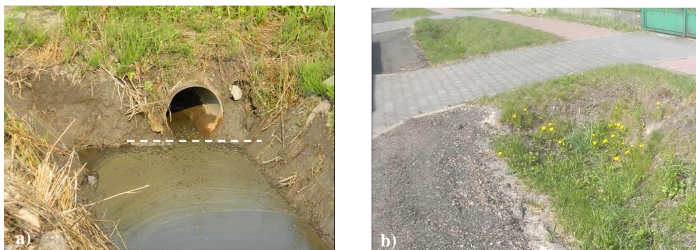
Fig. 3. Errors in the renovation of ditches: a) low ditch bottom, b) no culverts
