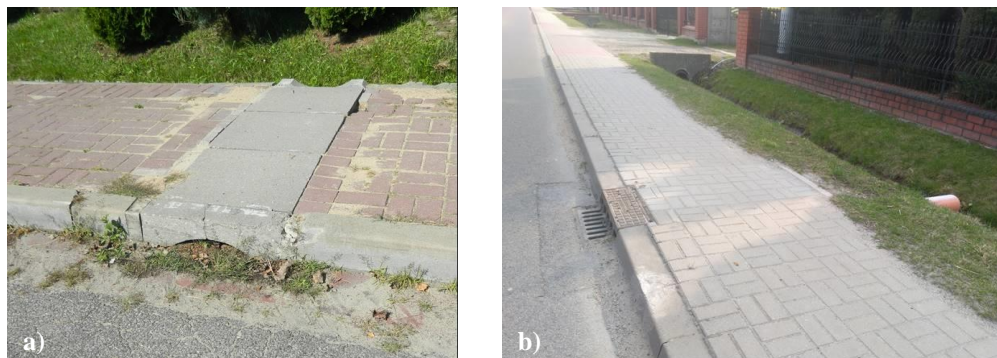
Fig. 4. Draining water with a conduit: a) cross-sections are too small, b) after replacement
