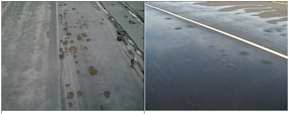
Fig. 1 Blisters containing gas on a) the waterproofing membrane b) the asphalt pavement
