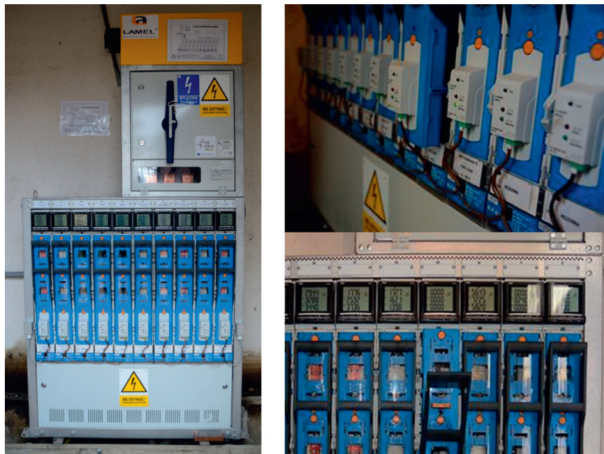
Photo 1. LV switchgear and controlgear assembly with individual LV circuits monitoring capability
