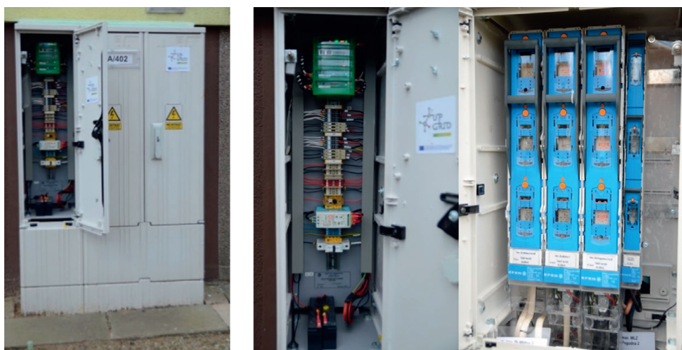
Photo 2. LV cable connectors with monitoring capability
