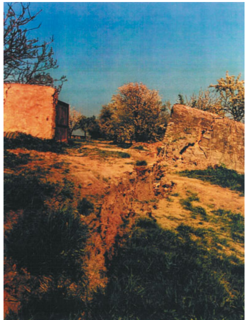
Photo 4. A view on the fractures and wall around the monastery
