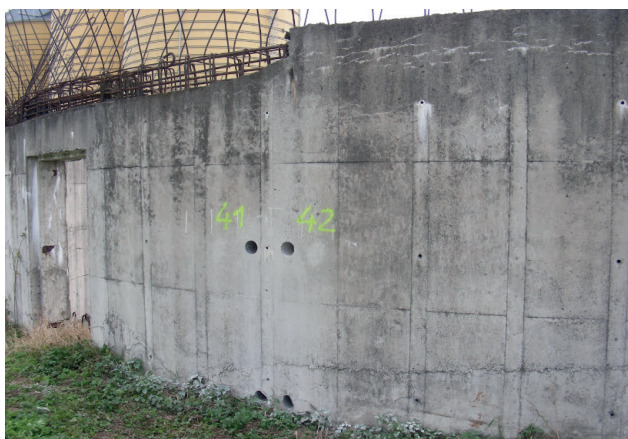
Fig. 5. Fragment of foundation No. 7 – visible salinity in concrete cracks, exposed corroded reinforcing bars and a trace of a break in concreting: no bonding of concrete placed earlier (lower) with concrete placed later. Darker color of the concrete surface. Degraded upper surface of the foundation wall
