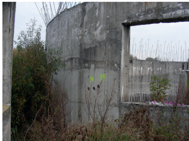
Fig. 3. Fragment of foundation No. 6. On the left, a narrow fragment of foundation No. 7
