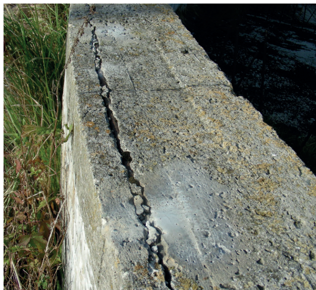
Fig. 7. Concrete delamination along a corroded reinforcing bar
