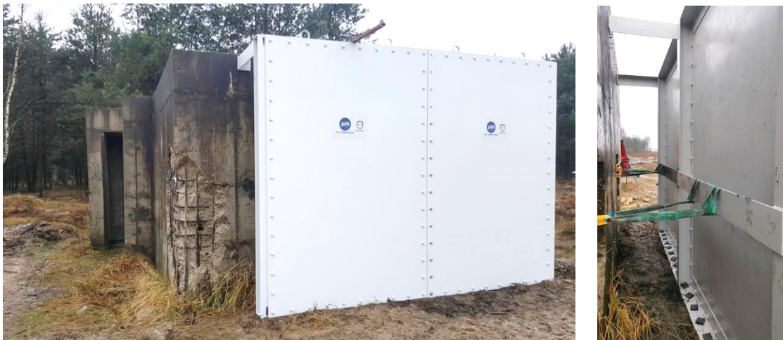
Fot. 4 i 5. Zamocowanie fasady na bunkrze Photo 4 and 5. Fixing the facade to the bunker
