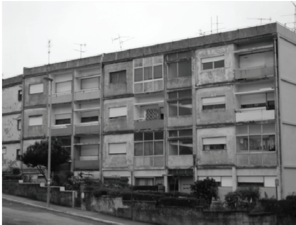
Fig. 5. Portuguese Building Needing Exterior Walls and Window Frames Rehabilitation
