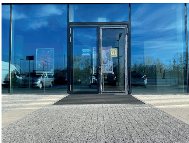
Fig. 22. An example of the correct transition between pavement types at the approach to building and the correct installation of an outdoor entrance doormat flush with the sidewalk surface. Opole. Toyota Park. Photo: M. Wijas
