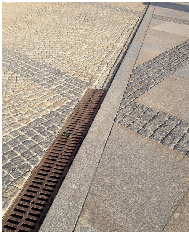
Fig. 3. Obstacle in the form of a drainage gutter installed below the pavement level, thus creating a ridge. Kielce. Photo: M. Wijas
