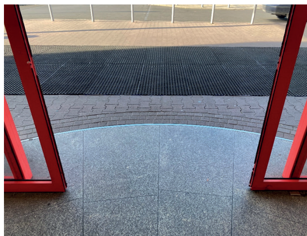
Fig. 23. A correctly installed door sill at the entrance to a shopping mall. Opole. Photo: M. Wijas
