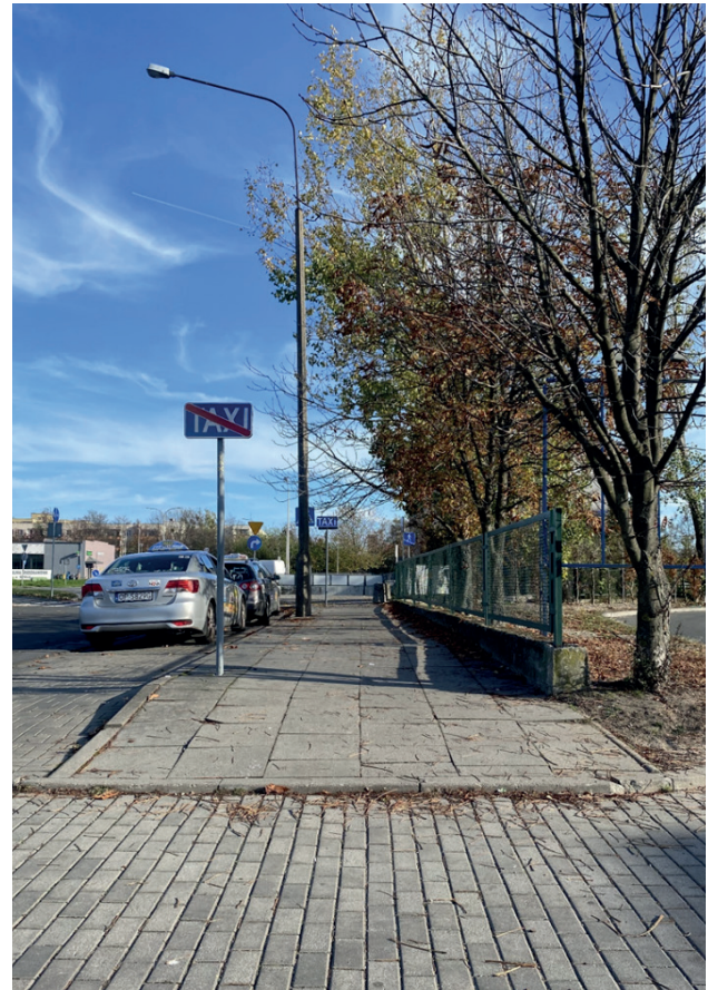
Fig. 17. An incorrect transition between a carriageway and a sidewalk. Obstacle in the form of a ridge of the height of more than 2 cm. Opole. Photo: M. Wijas
