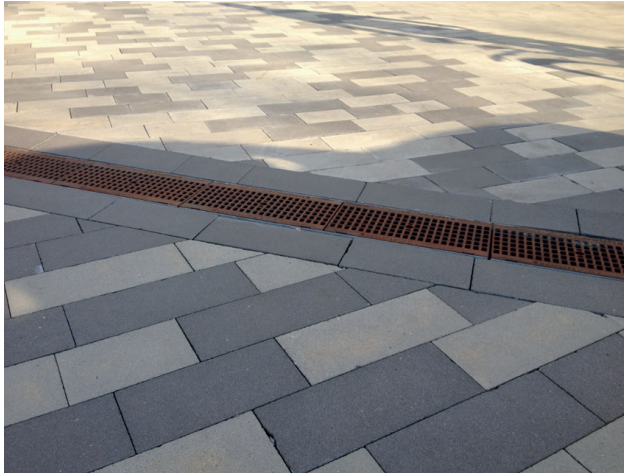
Fig. 4. A correct solution of a drainage gutter, which has been installed flush with the pavement of a shared zone. Photo: M. Wijas
