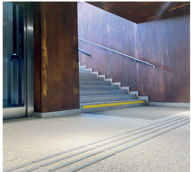
Fig. 5. An example of the correct yellow marking of staircase steps. Bus terminal. Kielce. Photo: M. Wijas
