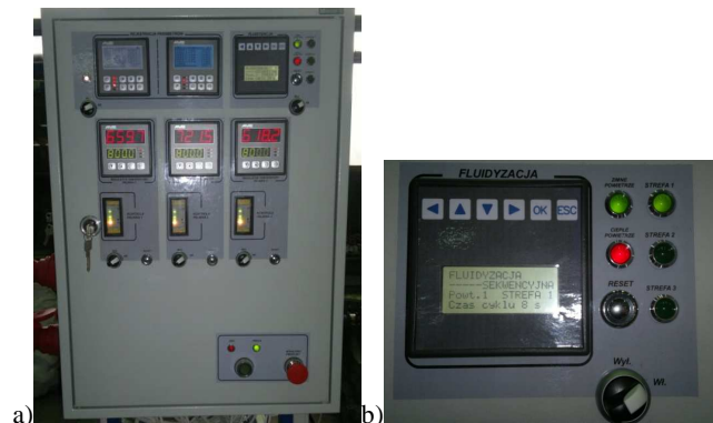
Fig. 3. System of controlling and recording operations of the thermal reclaimer a) General view, b) Control module of the fluidisation (bed mixing)
