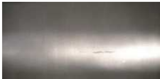
Fig. 1. The steel plate with a surface crack
