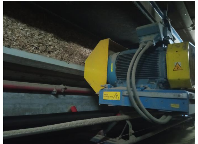
Fig. 2. Apparatus where the screw Conveyor is operating.
