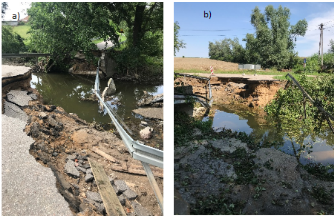
Figure 3. Crossing after the failure of the road bridge in Szeligi town.
