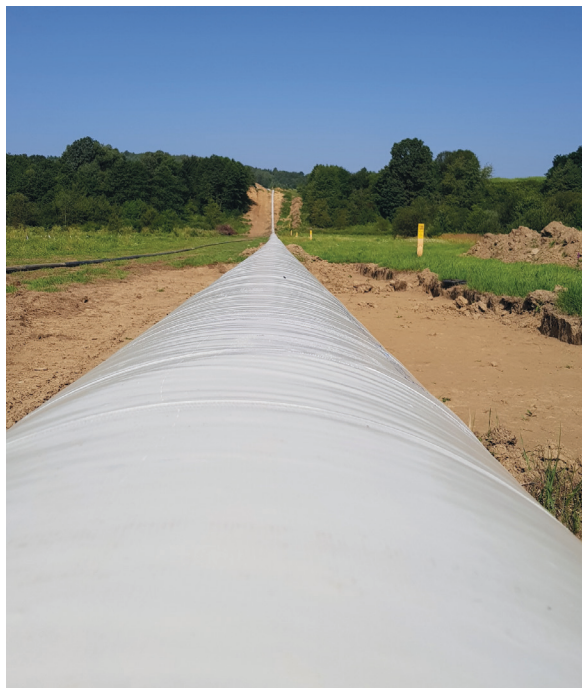
Fig. 3. Welded pipeline DN 700 979 m long with a protective layer [collection of J. Janicki]
