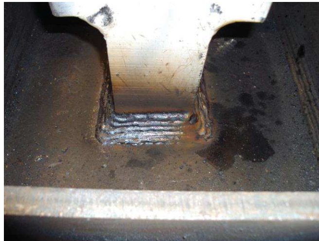
Fig. 3. Weld connecting the base of tilt cylinder's lifting eye fixation system with a gob shield top plate [12]
