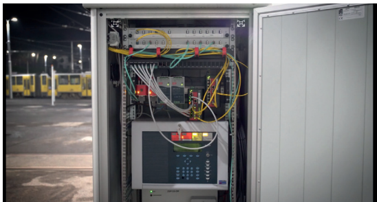
Fig. 2. Box with automatics and network devices on field [own study]
