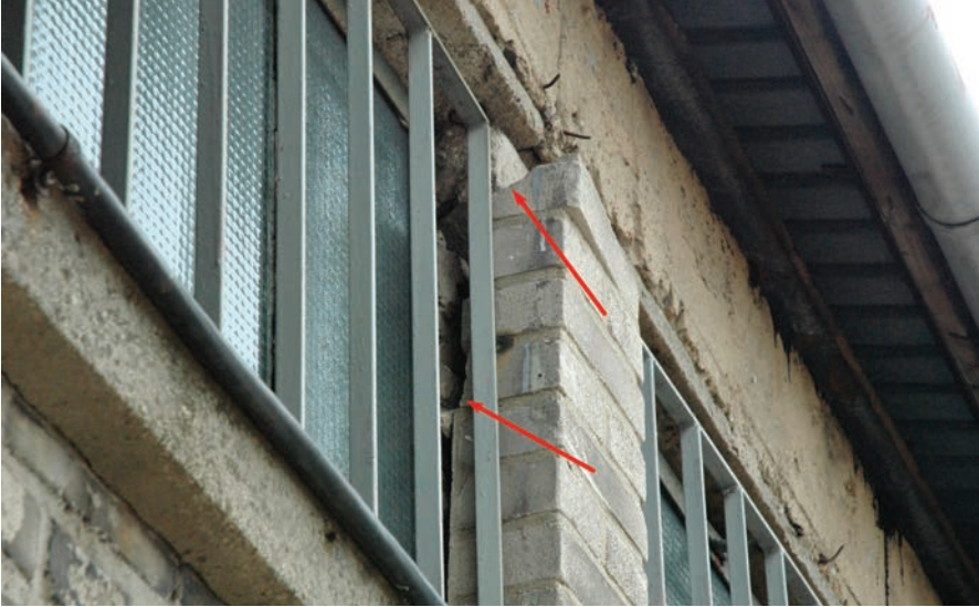
Fig. 9. Detail of the west elevation in the middle part – crack, displacement and delamination of a part of the brick pillar between the window openings
