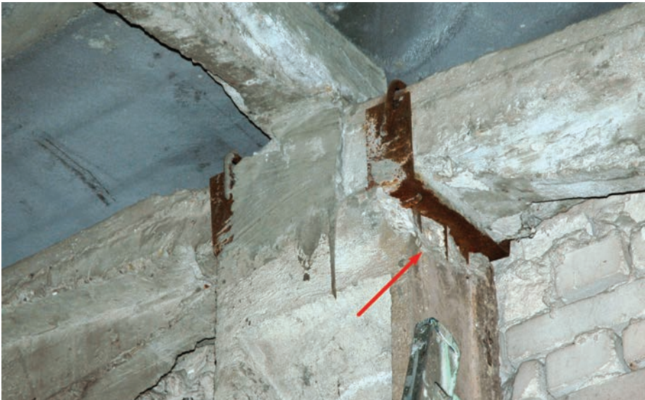
Fig. 2. The head of the central row column at the southern end wall. Loss of concrete of the depth up to 4 cm along the edge of the column head, at the level of the girder support
