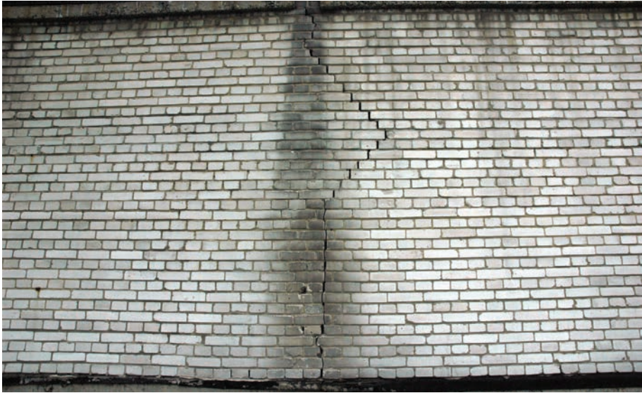
Fig. 4. Detail of the east elevation in the middle part – wall crack (up to 7 mm) in the vicinity of the load-bearing structure column
