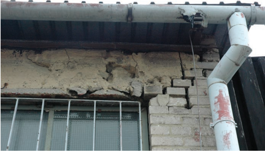
Fig. 10. Detail of the west elevation at the south corner – corrosion and delamination of the brick pillar as well as corrosion and cracking of the reinforced concrete lintel
