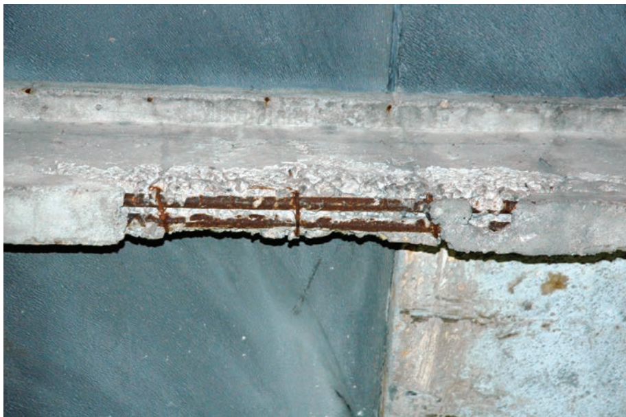
Fig. 3. The purlin in the middle part of the warehouse roof covering. Loss of concrete cover along the bottom edge of the beam and corrosion of the exposed rebars
