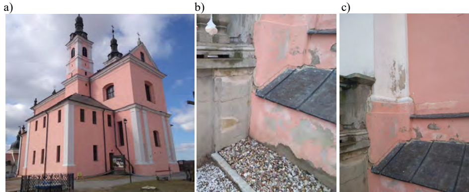
Fig. 3. A church under the invocation of St. Mary's Immaculate Conception - Wigry, a) general view of the building complex b) and c) visible outer layer damage caused by damp
