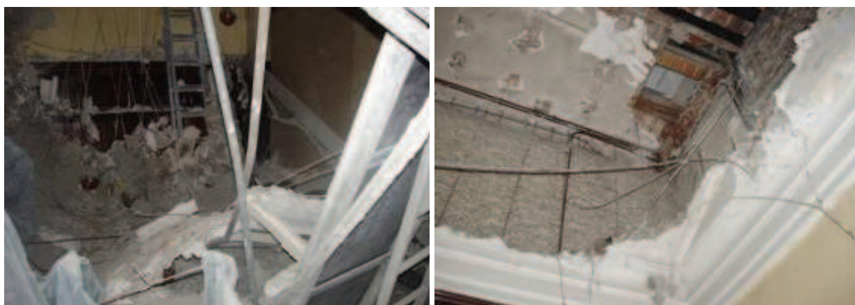
Rys. 8. Widoki zawalonego sklepienia Fig. 8. View of the collapsed vault
